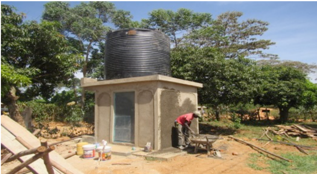
The water from this 10,000-liter plastic tank will supply the taps at the handwashing stations. The team worked with community members to complete this project.
